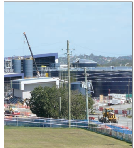
Tugun Desal plant
